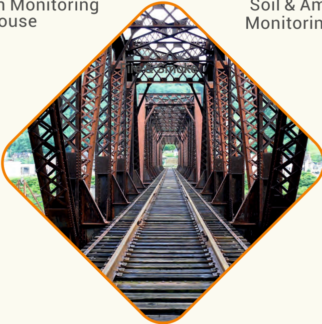
Vibes Span Structural Monitoring of Bridges
